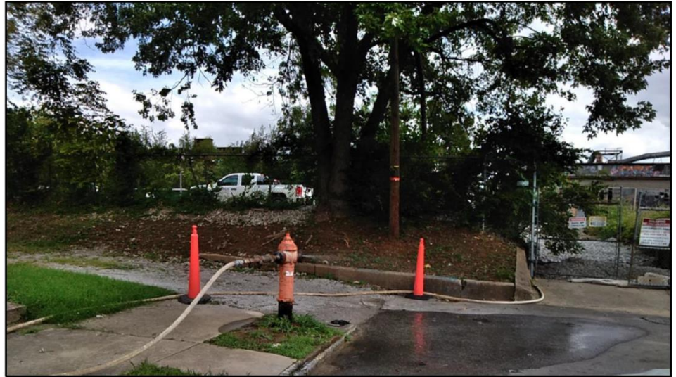
Black Leaf Chemical AI 52202 September 12, 2018 Photo of water connection in front of 1701 St. Louis Ave. Water is being used for dust/asbestos abatement. Air monitoring is also being conducted along the perimeter of the site on a routine basis for particulates, metals, pesticides, volatiles, etc.
