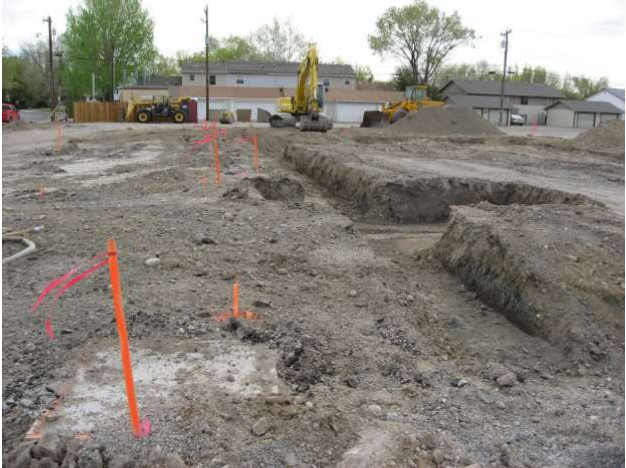
Figure 1 Trenching for AS/SVE system prior to restaurant construction. Remediation building is to the left behind the wooden fence.
