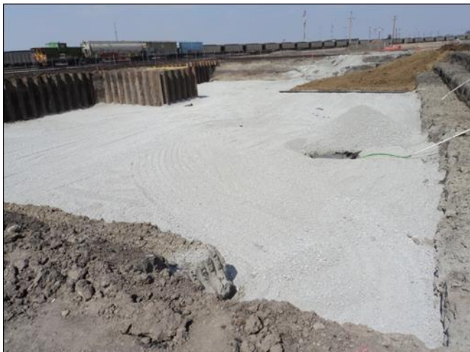
Excavation was backfilled with two feet of crushed rock and compacted soil to grade.
