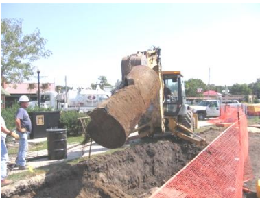
Discovery of an abandoned UST halts work on the new college campus.
