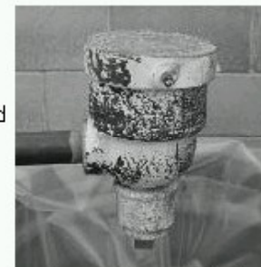
Source: Minnesota Dept. of Health, (mercury-containing device found on a low pressure system)
