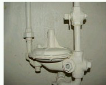
Source: Minnesota Dept. of Health, (disc-shaped mercury-containing gas pressure regulator)
